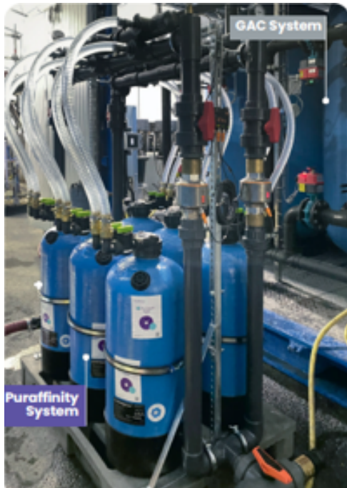
Figure 2: Puraffinity PFAS system (200L of media) which replaced a 4,000L GAC system.
