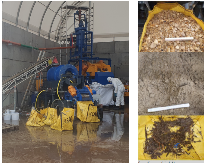
Fig. 2: PFAS soil washing pilot plant (left), washing fractions (right)
